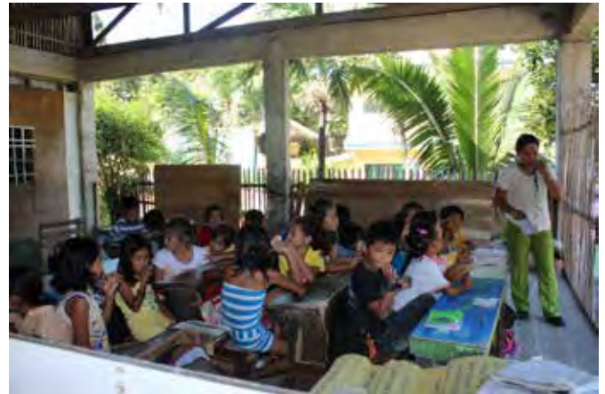
School resumed without repairing walls or windows
